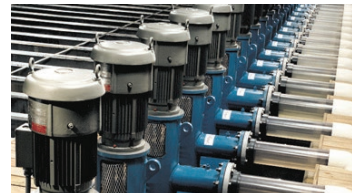
Vertical Pump in Operation
